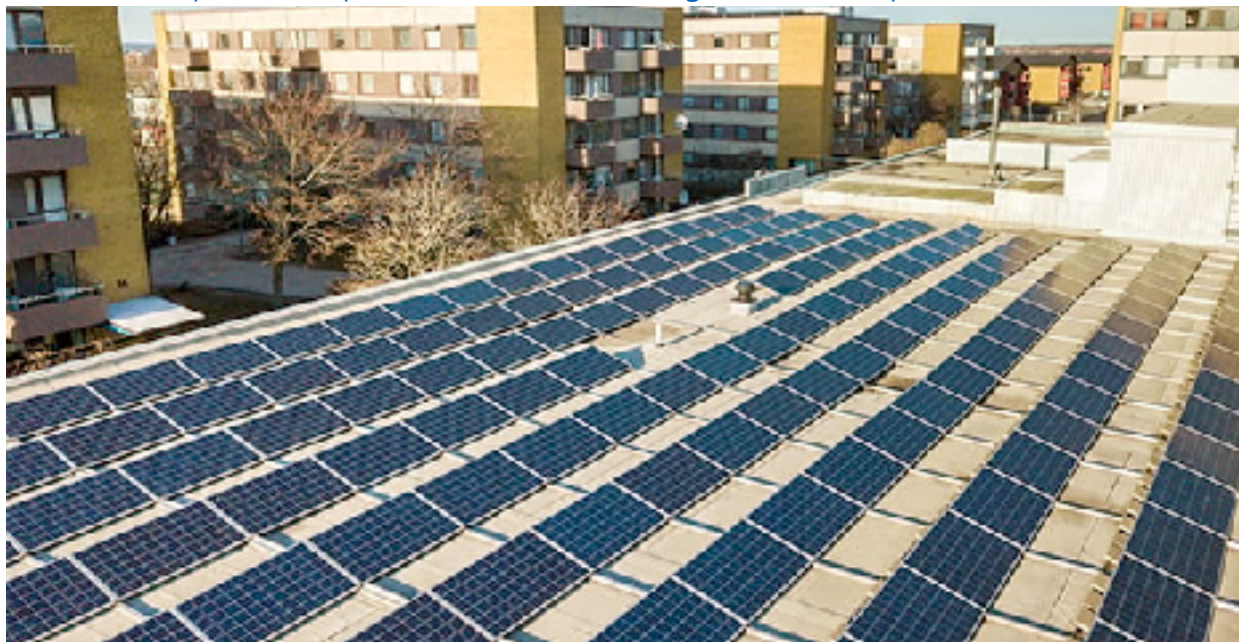
Exemple de tratări cu panouri fotovoltaice a acoperișurilor. Sursa: https://www.globest.com/2020/10/26/increase-your-assets-noi-with-solar-rooftop-tenants/?slreturn=20231104062956
