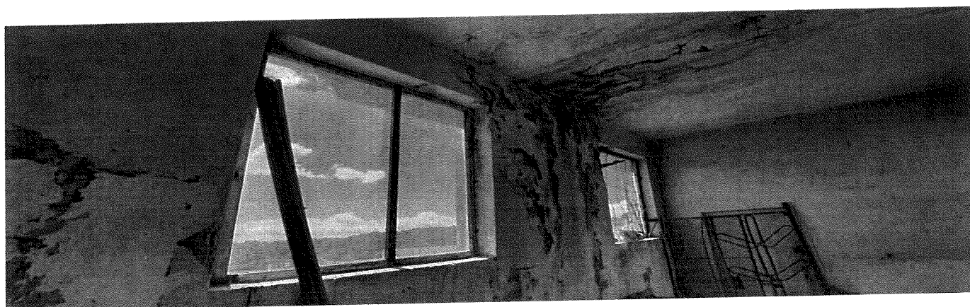
Infiltratii casa lift – acces terasa
