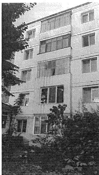
Inchideri balcoane fatada principala neconforme
